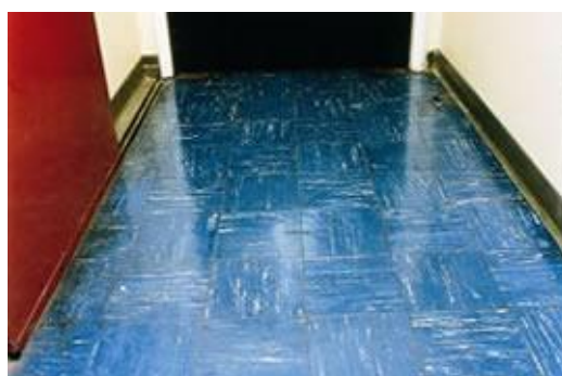
Asbestos containing floor tiles in a corridor
