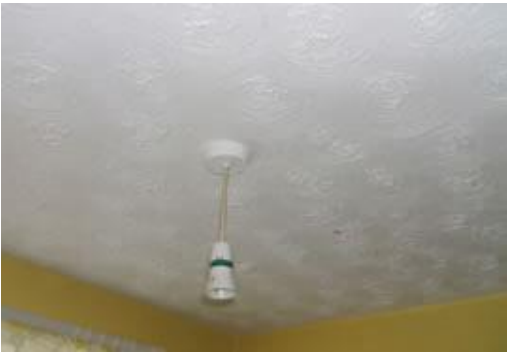
Asbestos textured coating
