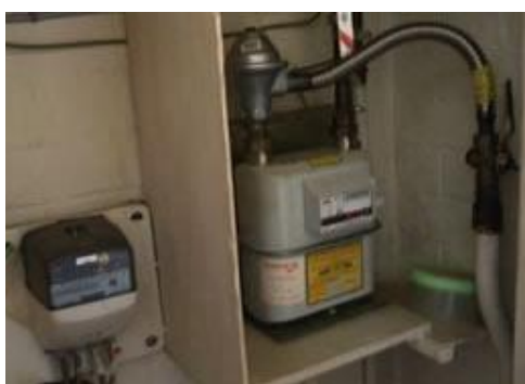
Asbestos panelling around a gas meter
